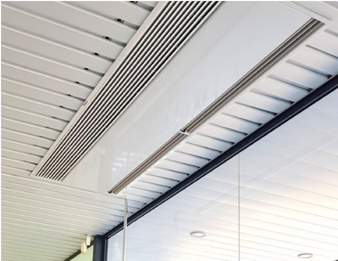
Recessed Windbox Integration in false ceiling in a shopping center
